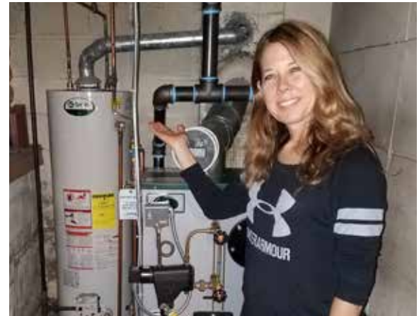
Heather McMahon's new boiler is just what this single mother of two needs before the winter heating season.
